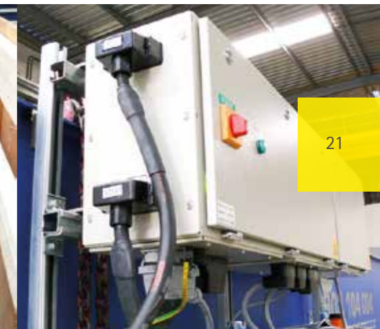
Bridge panel with plugs
